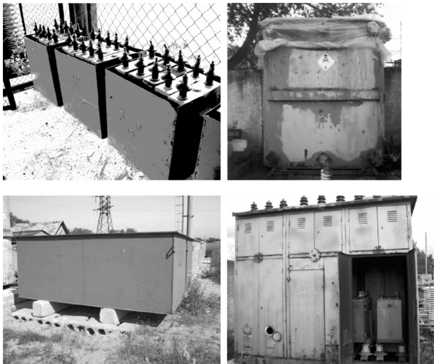
Figure 4. Types of containers for PCB-containing capacitors storage
